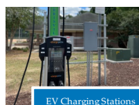
EV Charging Stations
